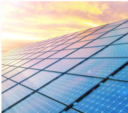
Solar Array Testing
